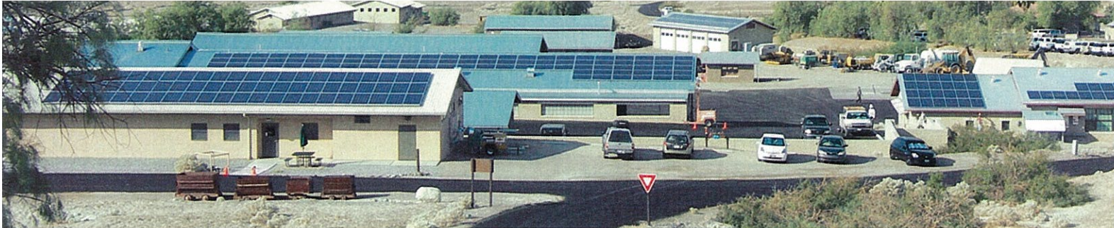
Photovoltaic system, Death Valley National Park, NPS Photo
